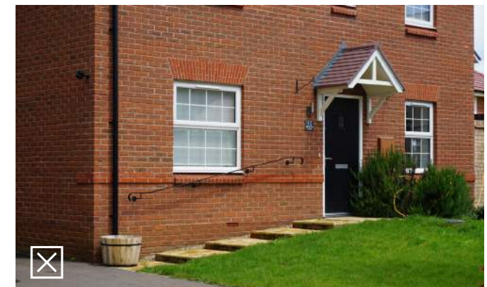
Access to property is made difficult by poor response to site levels
